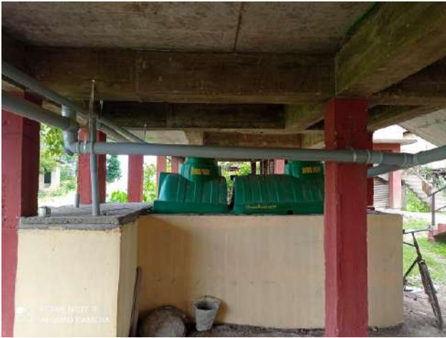
Septic Tank for indoor sanitation
